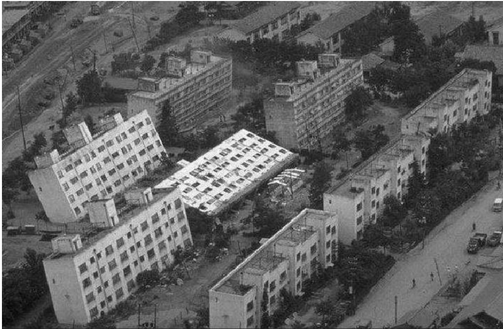
Figure 1. Overturning Failure of Apartment Complex Buildings During Niigata 1964 Earthquake (Courtesy of USGS) (Jakka, R.S. 2013).
