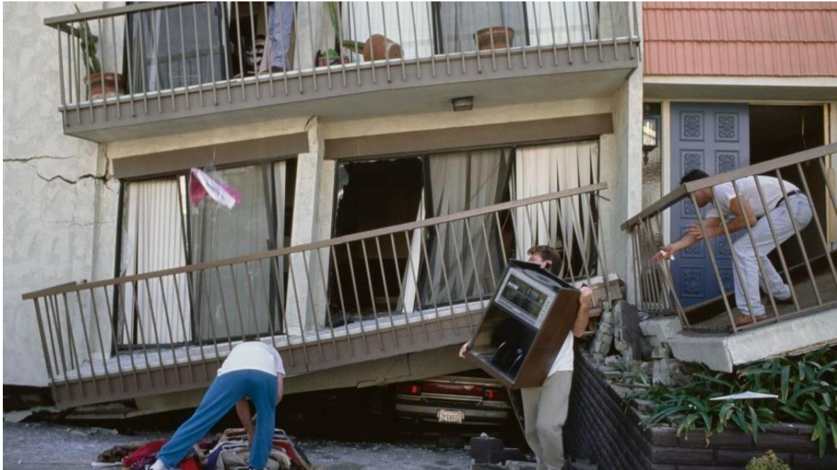
Figure 7. Consol Damage in 1994 Northridge Earthquake (Url 4)
