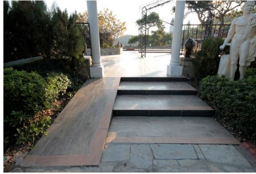
Figure V. The exterior ramp of Tekirova Corinthia Hotel is unexpectedly interrupted by a pillar; also tiled buffers should be installed to protect against possible sliding.
