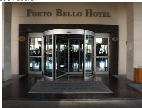
Figure III. Entrance door and the step is not supported by a ramp, Revolving doors obstruct the entrance for PwD, so alternative wide doors that are opened at 90° must be installed (Porto Bello Hotel, Antalya).
