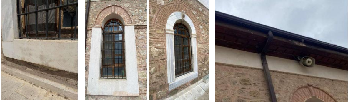
Figure 6. Material deterioration observed on auxiliary elements (Özçelik, Z. S., 2026)
