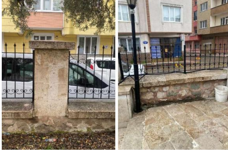
Figure 5. Material deterioration observed on floors (Özçelik, Z. S., 2026)
