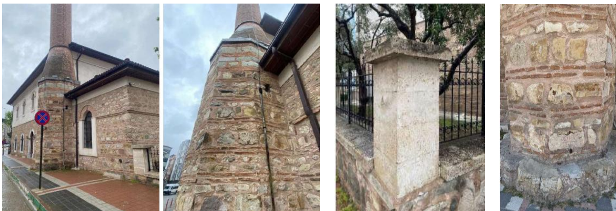
Figure 4. Material deterioration observed on walls (Özçelik, Z. S., 2026)
