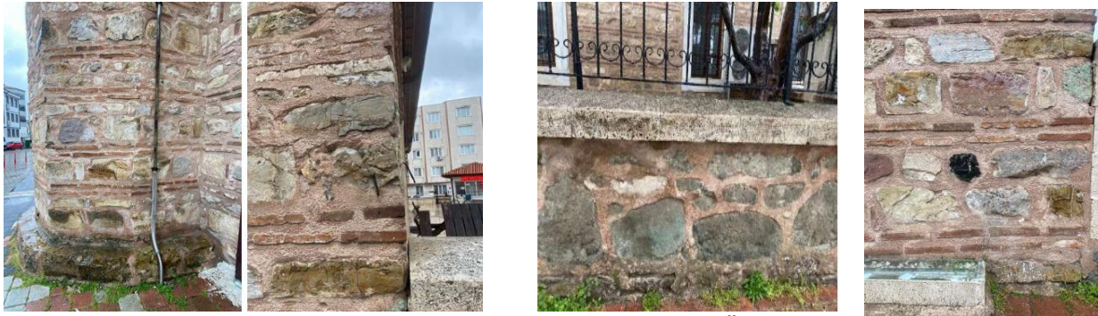
Figure 3. Material deterioration observed on walls (Özçelik, Z. S., 2026)
