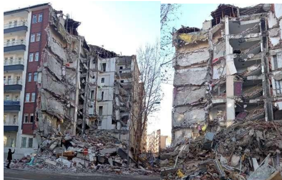
Figure 9: Insufficient design of structural elements
