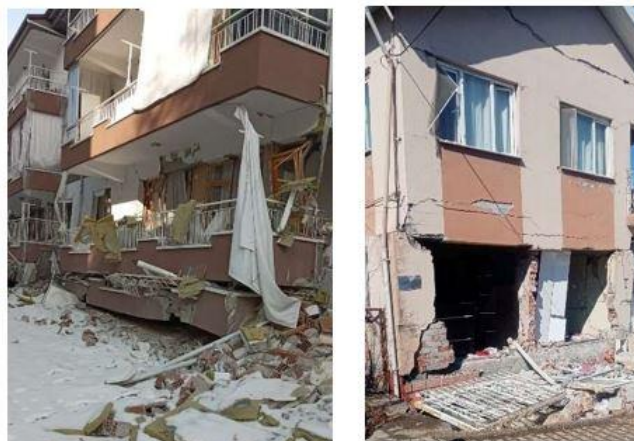
Figure 6: Weak storey damages in Malatya
