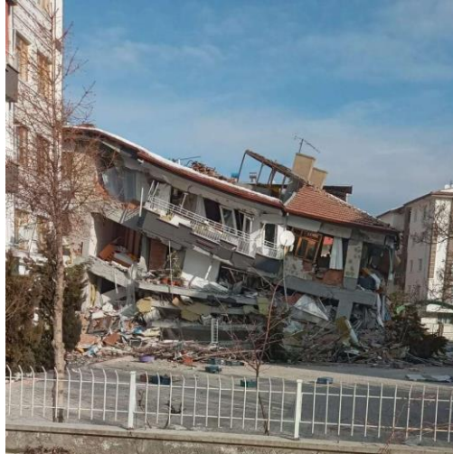
Figure 3: Torsional irregularity damages in Malatya
