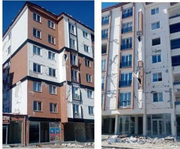
Figure 5: Projection damages in Malatya
