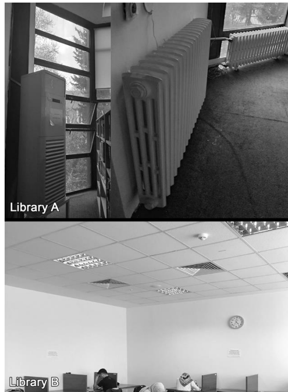
Figure 5. Heating and cooling systems
